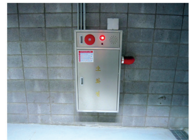
Firefighting Hydrant Systems
