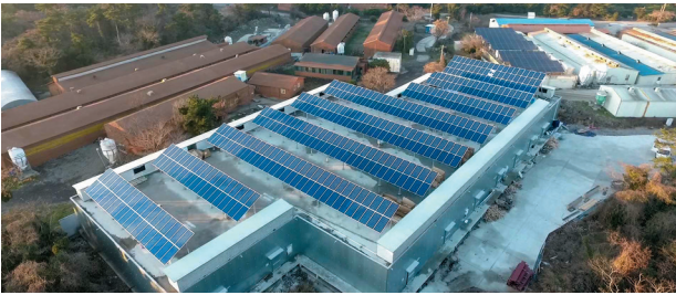
SM Solar Power Plant, Jeju
