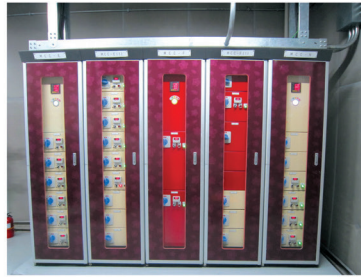
Firefighting MCC Panels
