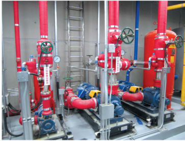
Fire Extinguishing Systems
