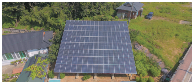
Jeongseok Solar Power Plant
