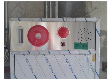
Firefighting Hydrant Systems
