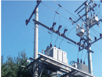
Power Receiving Equipment
